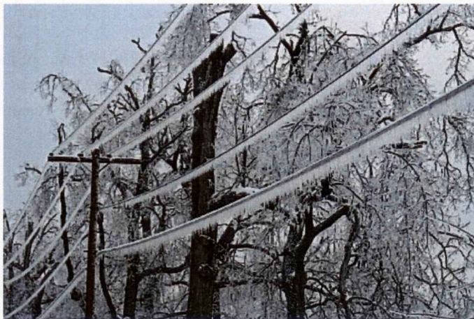
Figure 3-23 Ice Covered Power Lines
