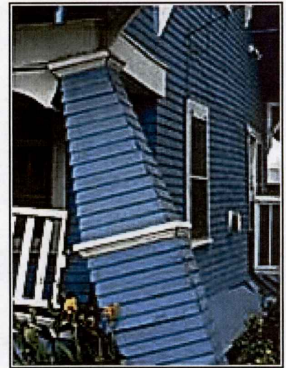
Figure 3-8 Earthquake Damaged Porch
